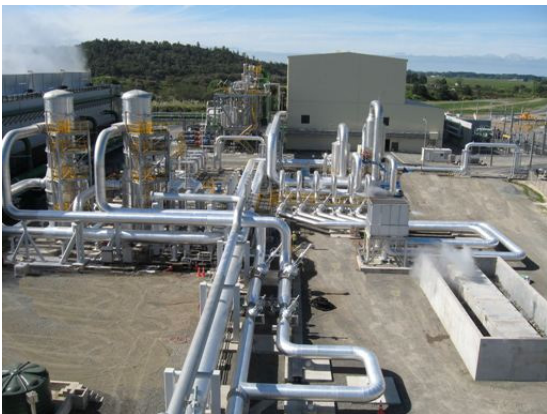
Figure 4: Photograph of Entire Power Station
