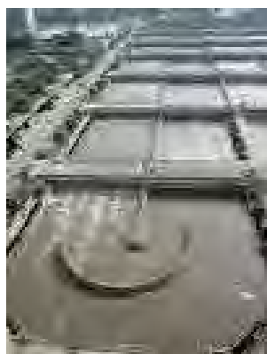
Figure 8.2.4 Large Scale OD Plant
