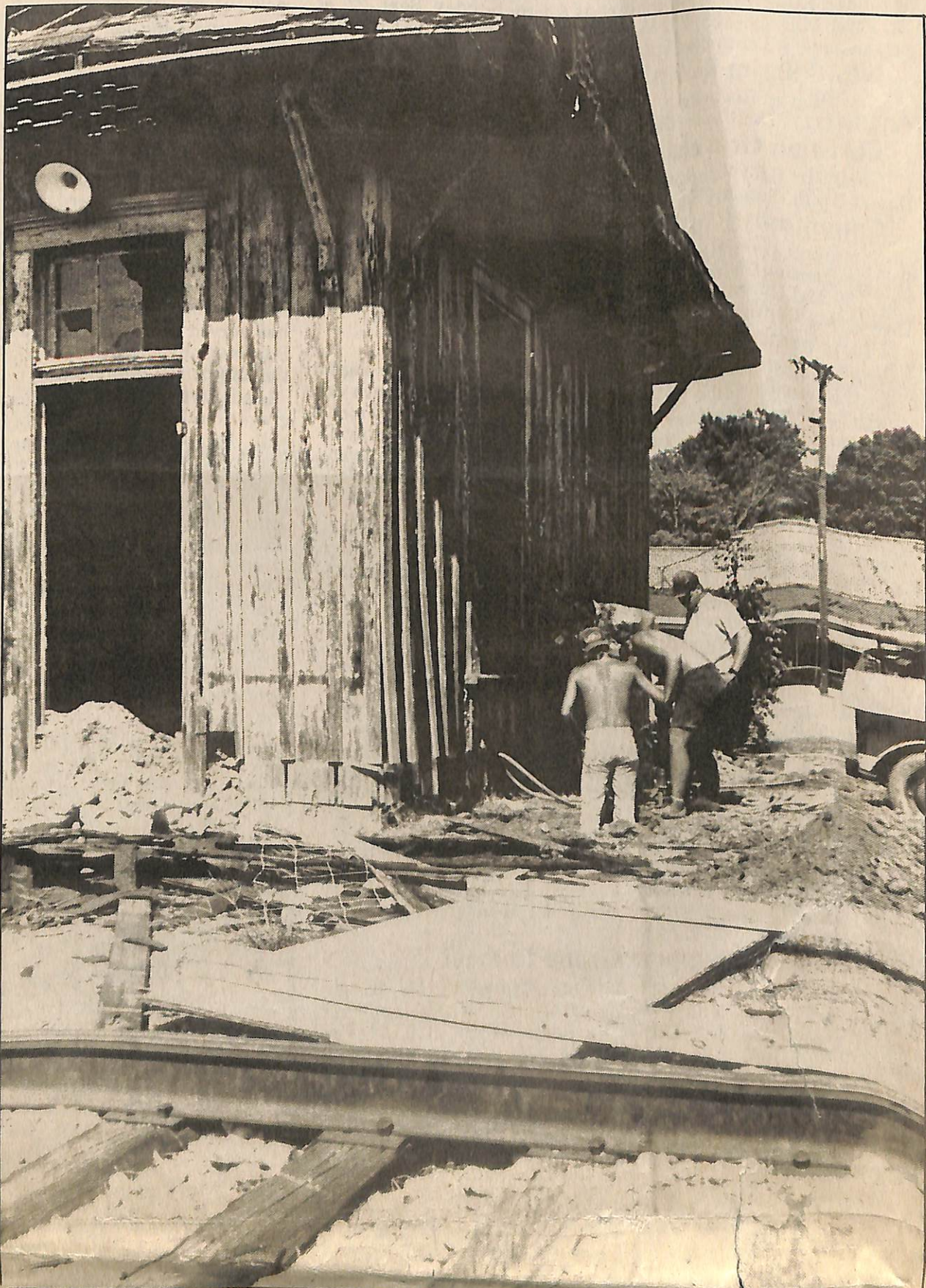
Workmen prepare Bentonia's turn of the century railroad depot to be moved
