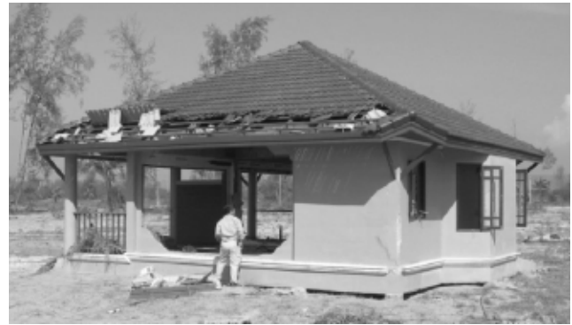
Photo 3. Damaged house by the tsunami at Ban Ma Kap.
