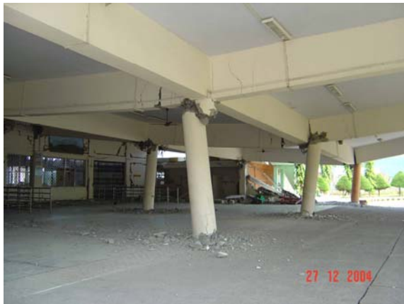
Fig. 2 - Damaged Passenger hall Building at Haddo Wharf, Port Blair, Andaman Island
