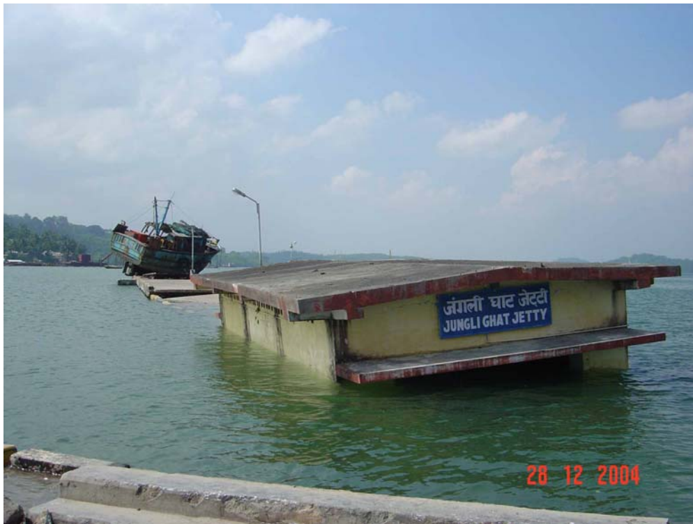
Fig. 5 Collapsed and submerged Jungali Ghat Jetty, Port Blair, Andaman Island
