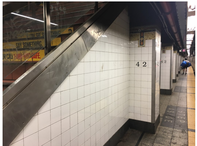
Northbound platform level looking north at stairway P15. Note the stairway bulk and tight clearance between the stair and the platform edge. This is typical of all of the original stairways on both platforms. Photo taken on the day of closure, May 31, 2018.
