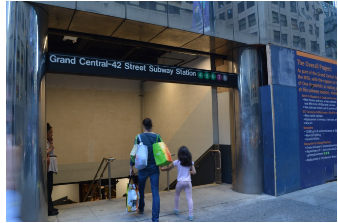
The street level opening of the reconstructed street stair within the Grand Hyatt Hotel building envelope on the west side of Lexington Avenue just north of E. 42 nd Street on June 15, 2018. A new ADA elevator is being built to the right.
