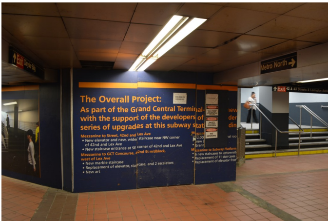
The mezzanine level landing of the new ADA elevator will be located directly behind this construction barrier, to the left of the rebuilt street stair. June 15, 2018.
