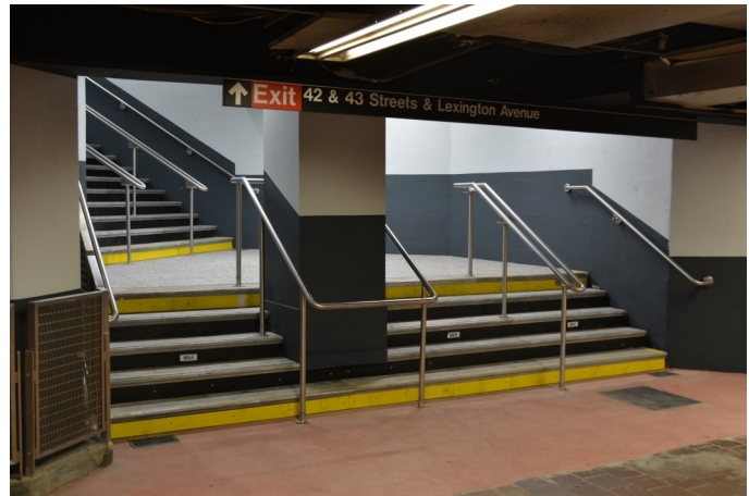
Reconstructed and widened street stairway from the north mezzanine to Lexington Avenue, one day after reopening on June 15, 2018.
