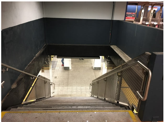
Looking down P24 on April 17, 2018. Note the narrower width of the new stair structure relative to the original opening.
