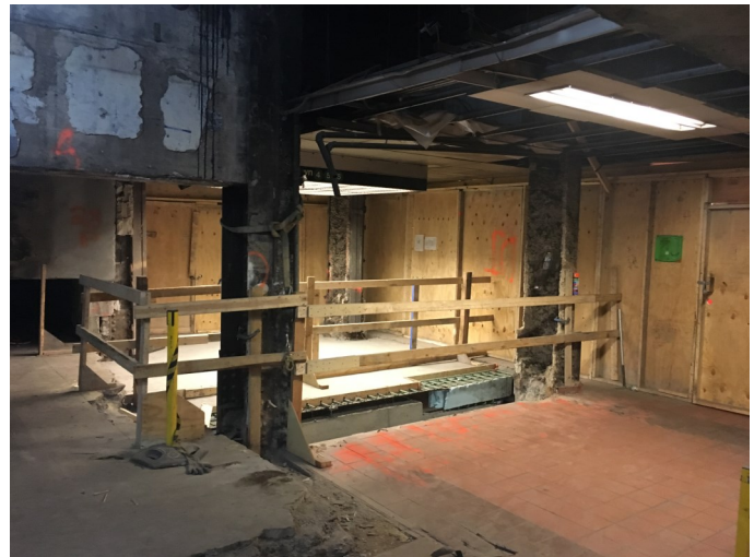
Behind the construction barrier on May 21, 2018, looking northeast at the space formerly occupied by P23. The stair was demolished and the void has been filled in. A new, repositioned P23 will be constructed to the right.
