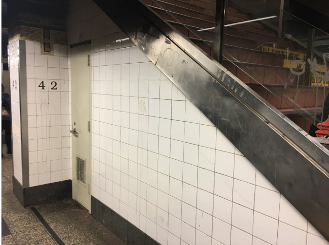
The ancillary support space underneath the P15 stairway structure will be relocated off the platform to free up space. May 31, 2018.
