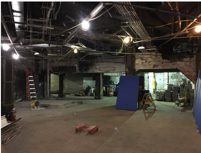
Former Grand Hyatt Hotel basement space, looking northwest, June 8, 2018. By late next year, this will be part of the new continuous mezzanine.
