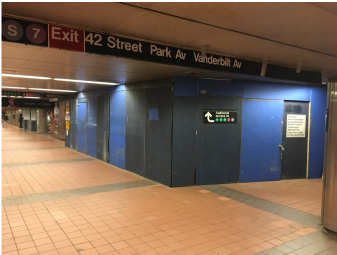
Mezzanine level, looking southwest. The construction barrier encloses the Grand Hyatt Hotel basement space. Stairway P23 to the northbound platform was previously located directly behind the construction barrier in the foreground, May 11, 2018.
