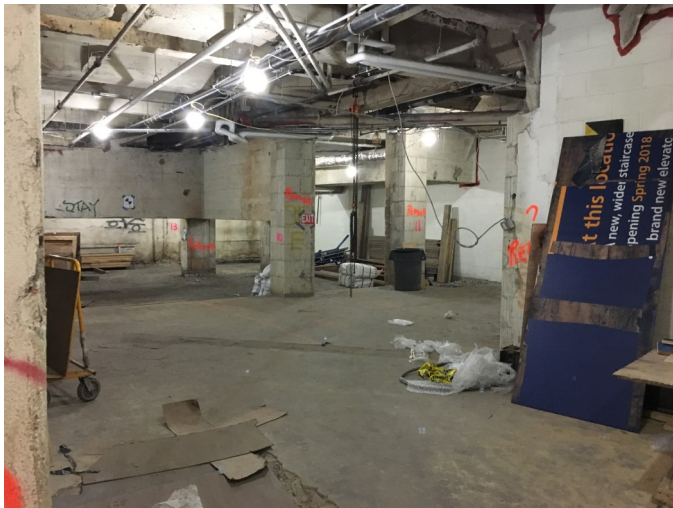
Another view of the northern basement space, looking north, on June 15, 2018. Two new stairways will be built from here to the north end of each platform.
