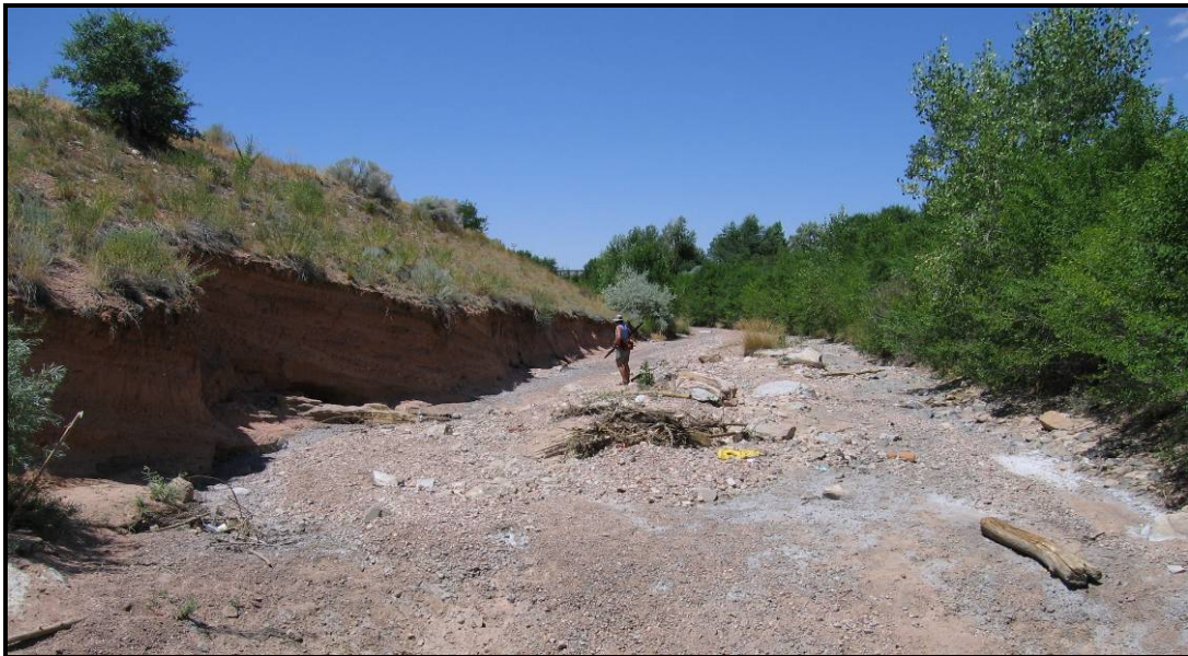
Figure 8.F. Undercut banks where design lacked reinforcement Photo facing downstream Source: photo by author (2005)
