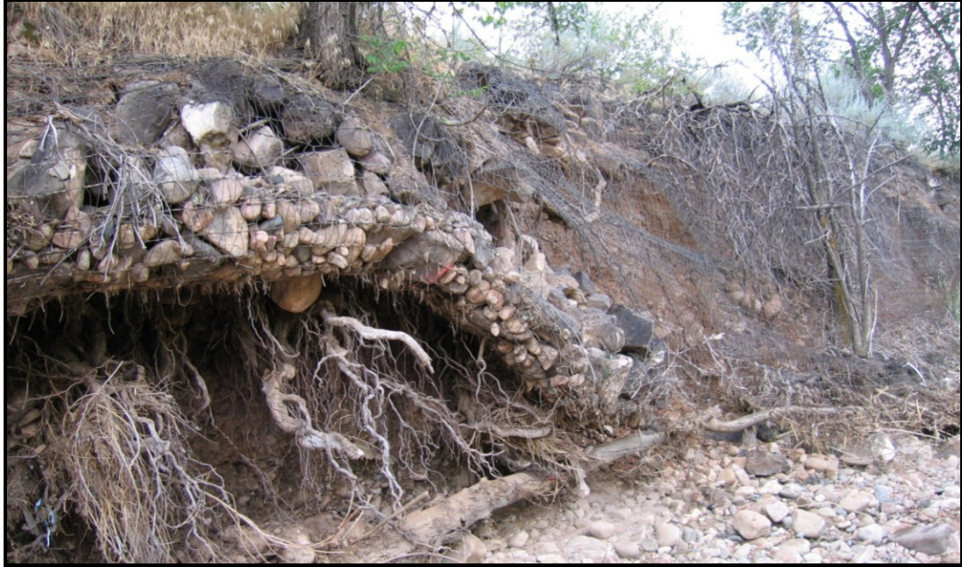
Figure 6.DD. Gabion failure from undercutting Photo facing downstream Source: photo by author (2005)
