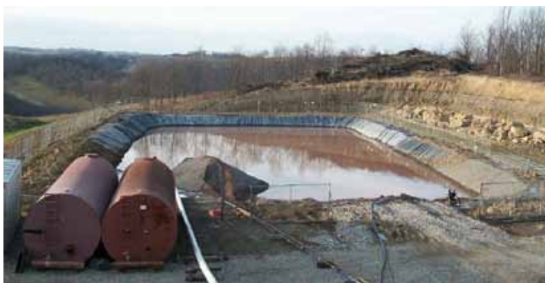
An on-site impoundment is one option for temporary fresh-water storage prior to fracking.
