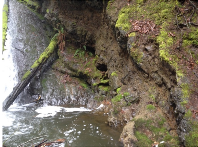
Photograph 4: View of north side of existing spillway chute from discharge pool at base looking upstream.
