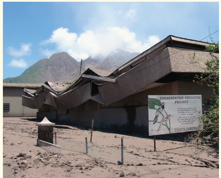
Roof collapse due to ash loading in Plymouth
