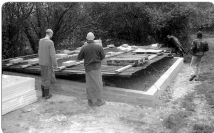
Ajahn Jutindharo, Ven Suvaco and Mouse survey the beginnings of the construction of the new workshop.
