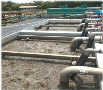
Membrane Bio Reactor
