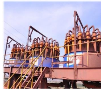
Slime Recovery Plant
