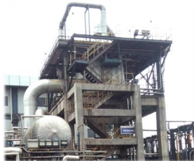
ZLD at Coke Oven
