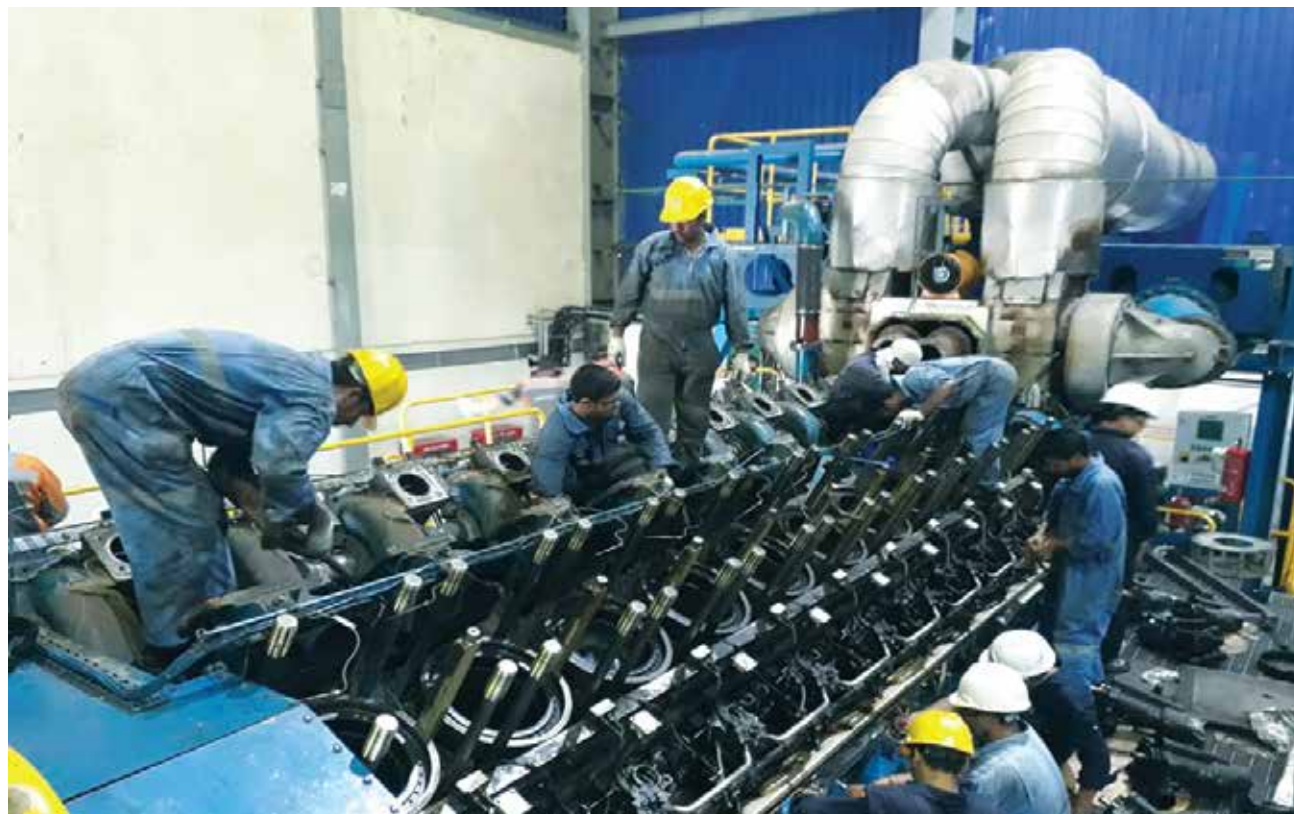
Major Inspection (MI) work of Raozan 25.50 MW Dual-Fuel Power Plant at Raozan, Chattogram.
