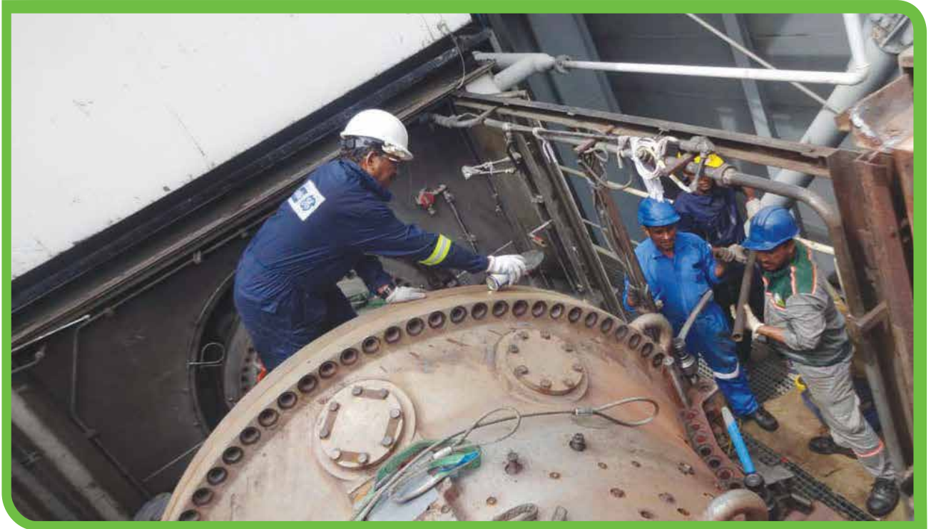
Major Inspection (MI) work of Gas Turbine of Mymensingh 210 MW Combined Cycle Power Station at Shambhuganj, Mymensingh.
