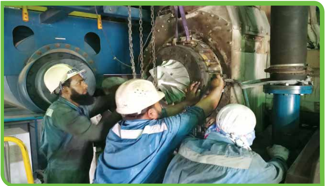
Major Inspection (MI) work of Gazipur 52 MW Dual Fuel Power Plant at Kadda, Gazipur.
