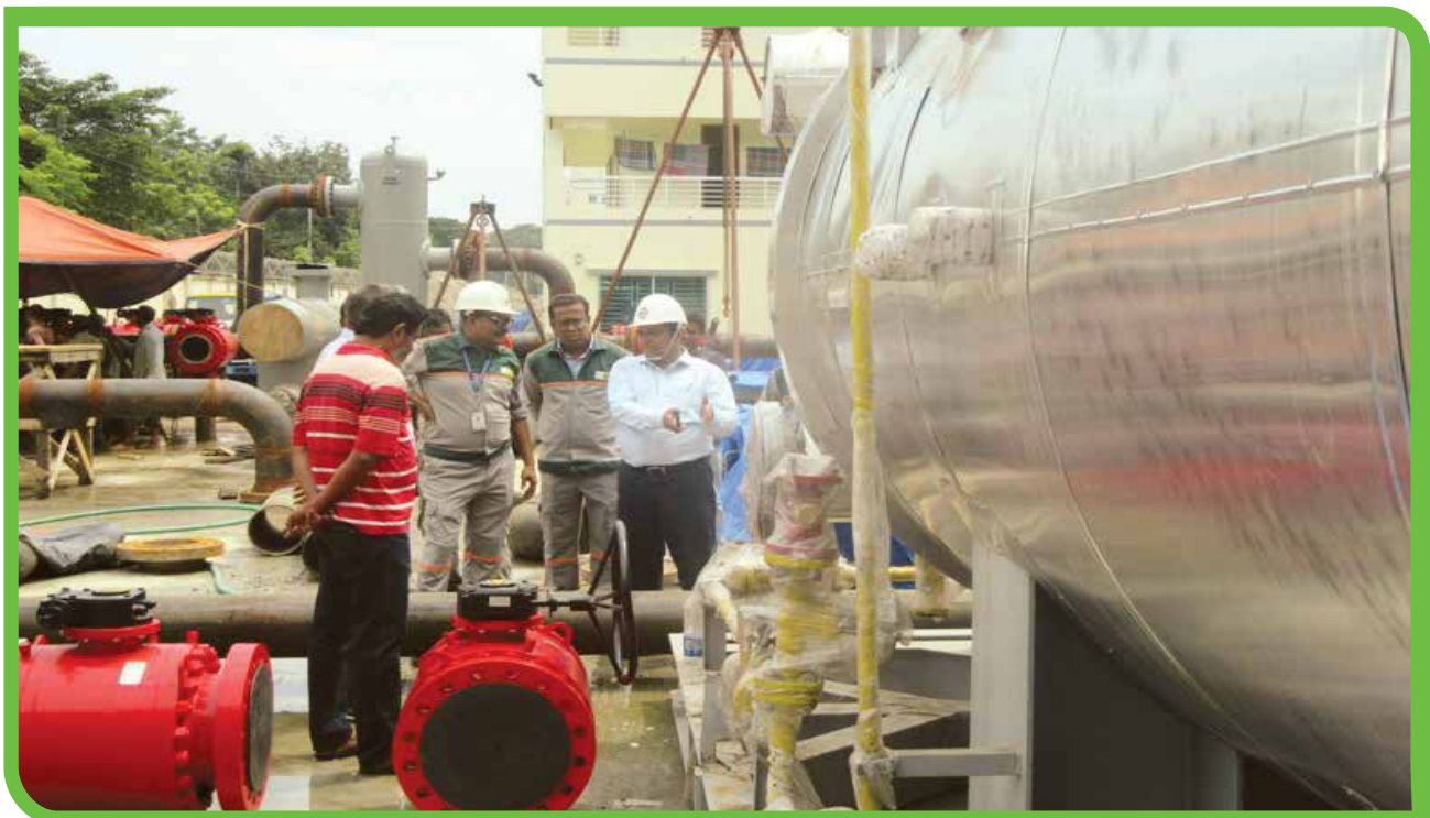
Inspection of newly Installed RMS Valve Station of Mymensingh 210 MW Combined Cycle Power Station at Shambhuganj, Mymensingh by Managing Director, RPCL.
