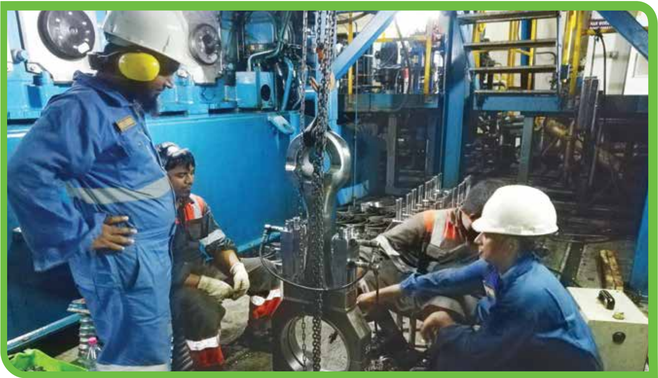
Major Inspection (MI) work of Raozan 25.50 MW Dual Fuel Power Plant at Raozan, Chattogram.
