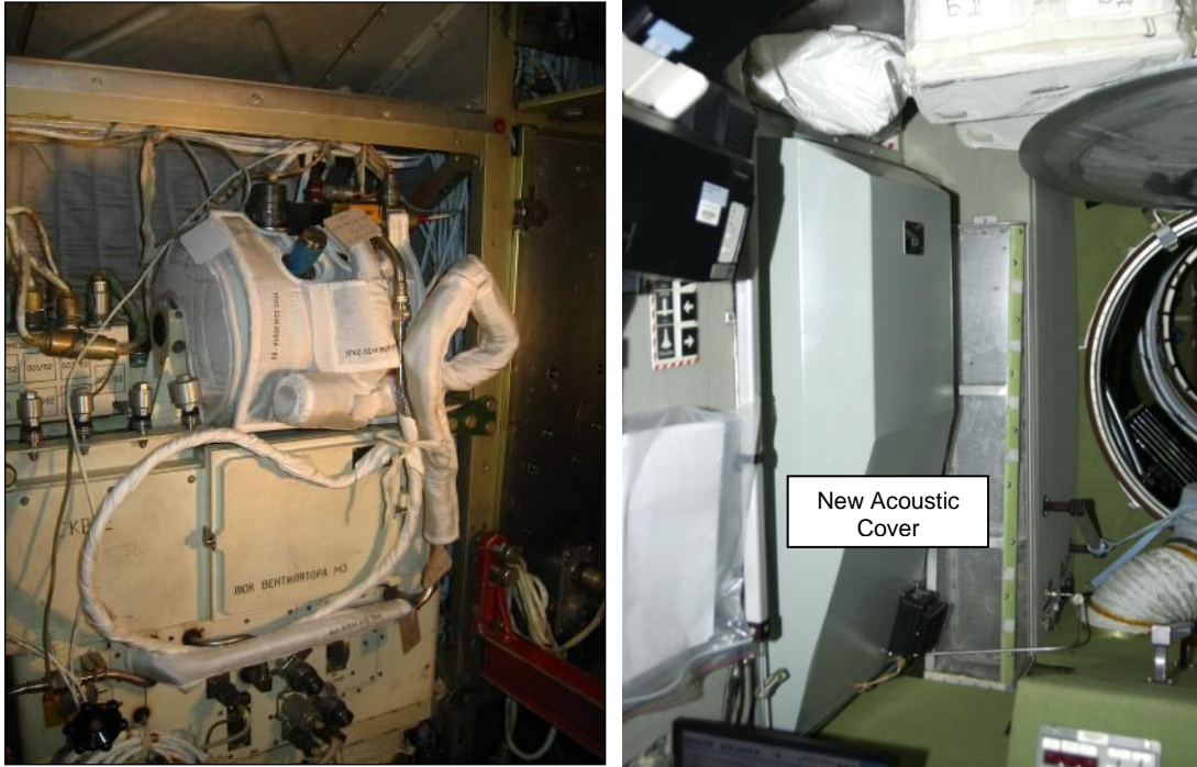
Figure 18. Air conditioner (CKB) acoustic treatments including compressor and fluid line wrappings (left), and the new single-piece acoustic close-out panel (right).
