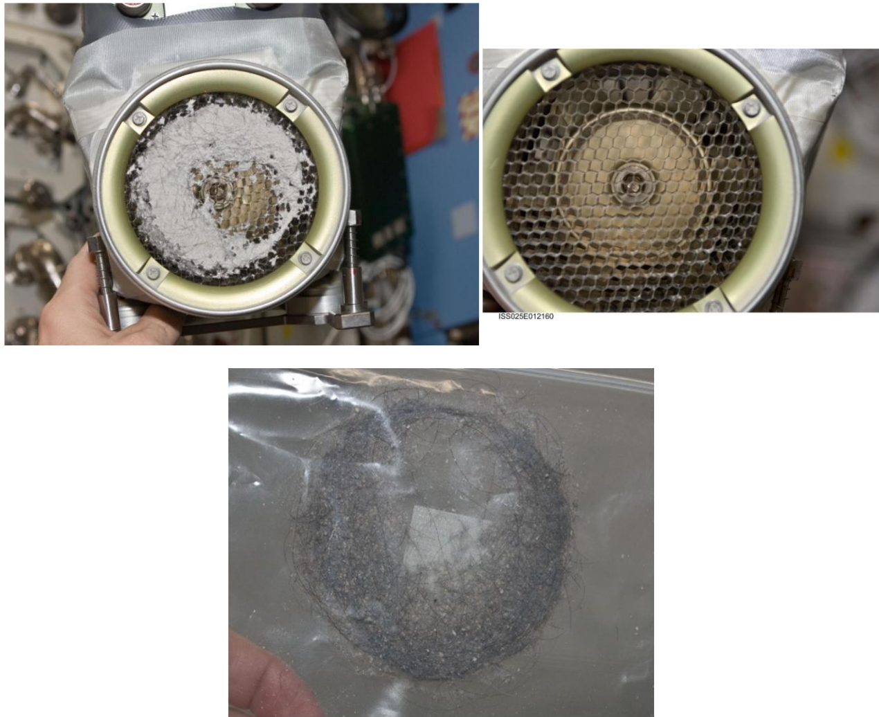
Figure 27. Clogged JPM IMV fan, before (upper left) and after (upper right) cleaning, dust removed is also shown (lower).
