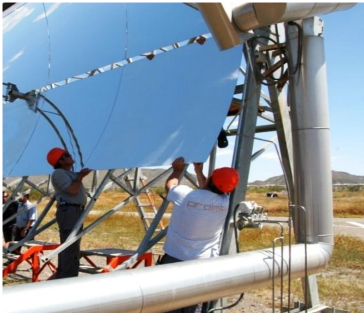
Figure 15: Mounting of a parabolic trough with silver coated glass mirror facets (source: CSP Services)
