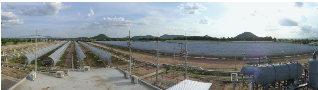
Figure 58: Kanchanaburi Solar Thermal Power Plant (source: Solarlite)
