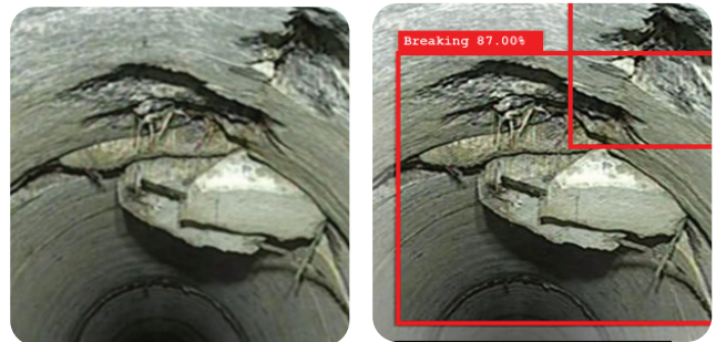
VAPAR's AI models process pipe inspection video footage to detect various issues in pipes. The issues found are then used to grade the pipe's health on a 1-5 scale. Image courtesy of VAPAR.
