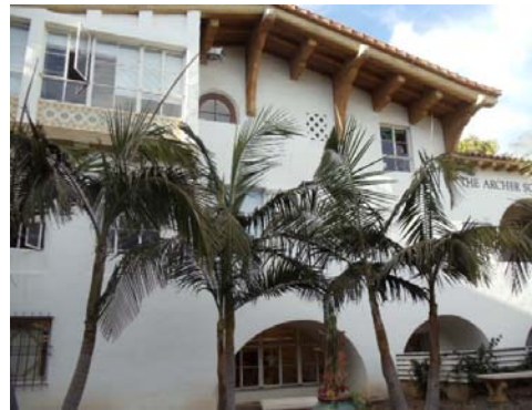
Detail of basement window wells and original second story steel casement windows, 2011. Source: Parallax Architecture and Planning.
