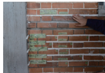
Mortar joint examination in progress at the former Tomioka Silk Mill (a Designated National Treasure)
