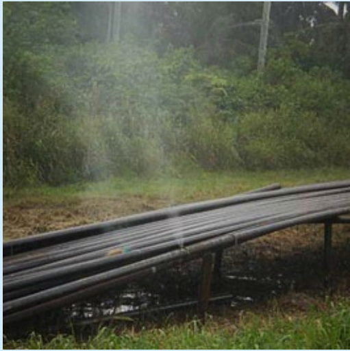
▲ Leaking Agip gas pipe in Ebocha community, Rivers State, Nigeria © ERA
