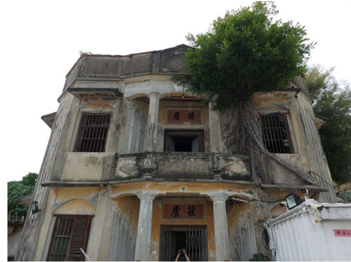
Figure 2. Existing undocumented trees on the external wall of Siu Lo
