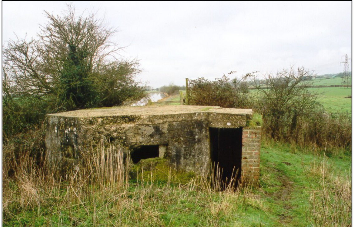
Fig. 12 - UORN 8223: type 22 pillbox dug into the rampart of the Royal Military Canal. The pillbox has sustained some damage to one of its faces and embrasures.
