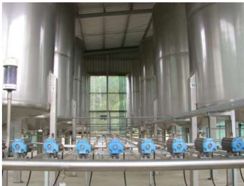
Figure 9.33. The ‘tank farm’ at the former ‘Maincamp’ Property (Photo courtesy of Mr. John Bax).
