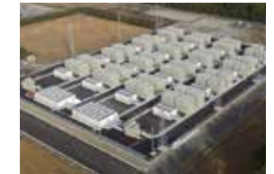
Buzen Battery Storage and Transformer Station
