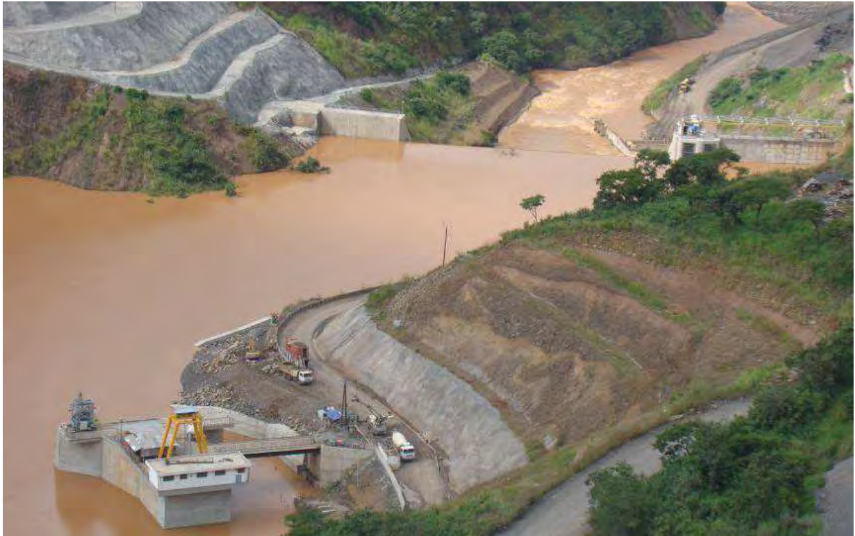
Figure II - 12: "Weir" on the Gilgel Gibe and slope stabilization Source: Salini photographic doc.
