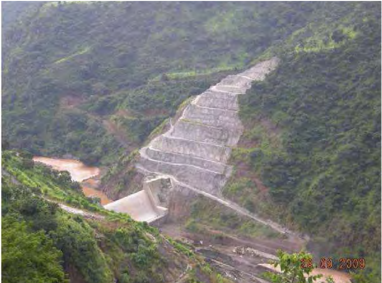
Figure III - 49: Shotcrete slope stabilisation on the mountainside to the left of the dam Source: ELC, October 2009
