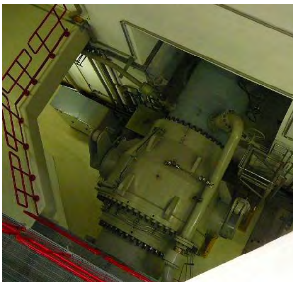
Figure II - 27: Main Inlet Valve
