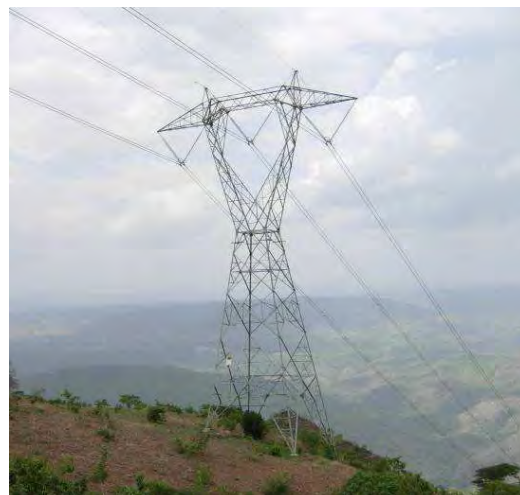
Figure III - 8: High voltage 400 kV pylon from GGII to GGI
