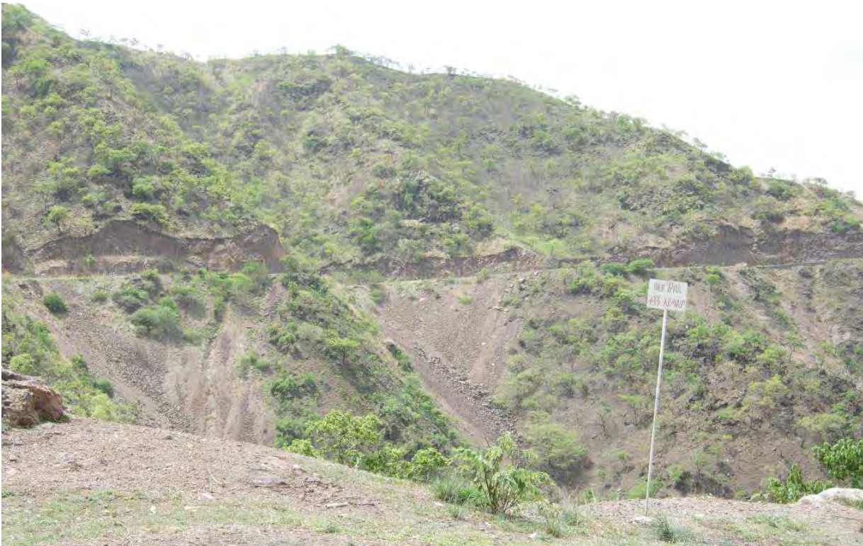
Figure III - 47: Stabilisation of slopes on the mountainside to the left of the dam Source photographic documentation of the evaluation team. 05.2012
