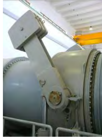
Figure II - 22: Penstock closing valve
