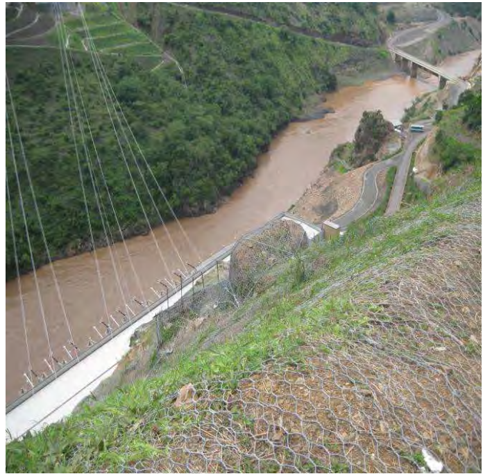
Figure III - 31: Mountainside stabilisation, Power H. area, using wire netting and riveting Source: General Contractor photographic doc., 08.2009
