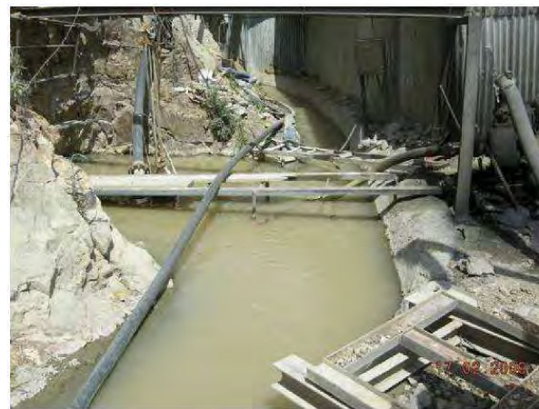
Figure III - 23: Waters discharged from the TBM excavation activity and dumped directly into the river without any processing Source: ELC, February 2009
