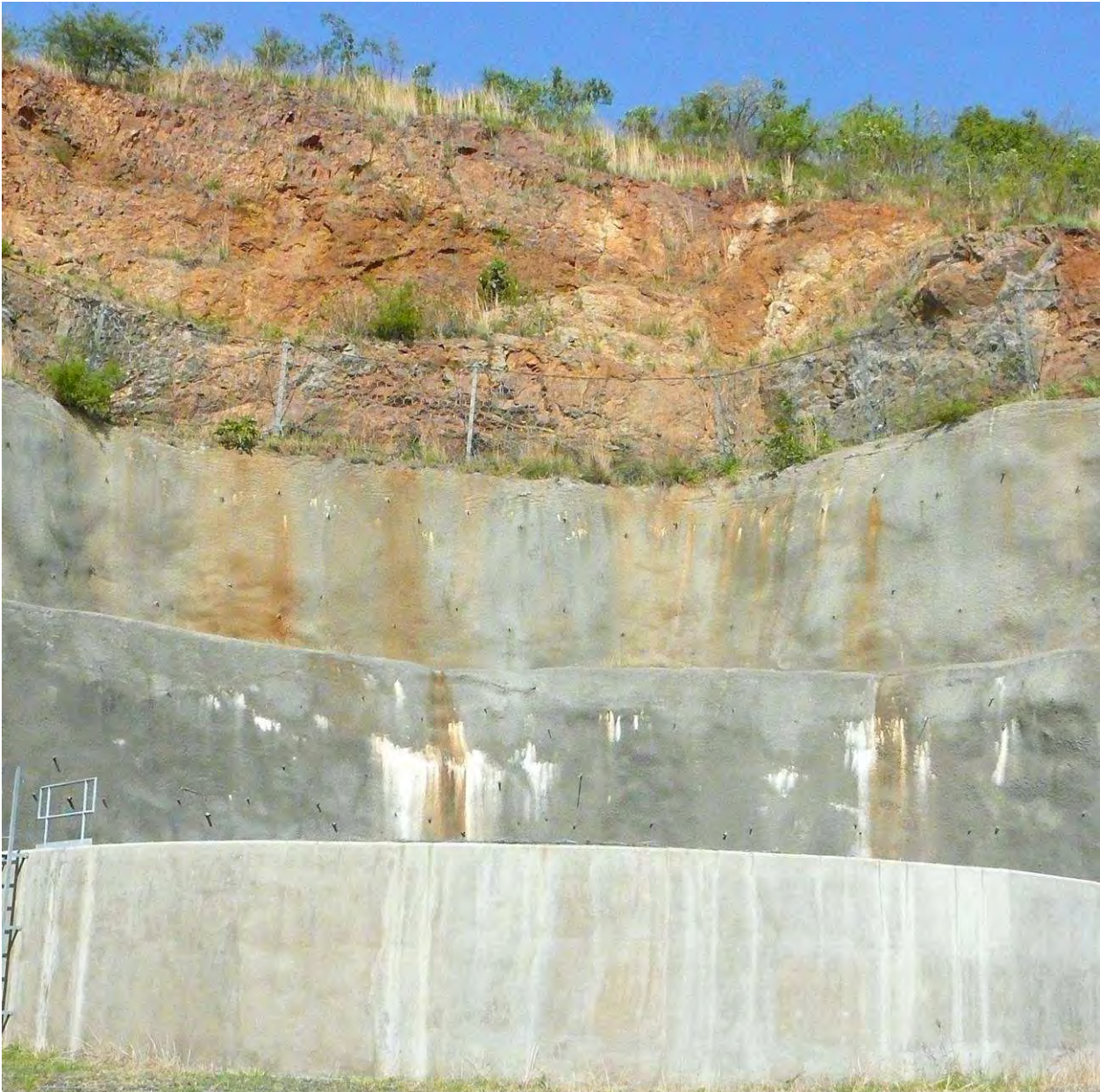
Figure II - 19: "Surge shaft" slope with salt incrustations Source: photographic documentation of the evaluation team
