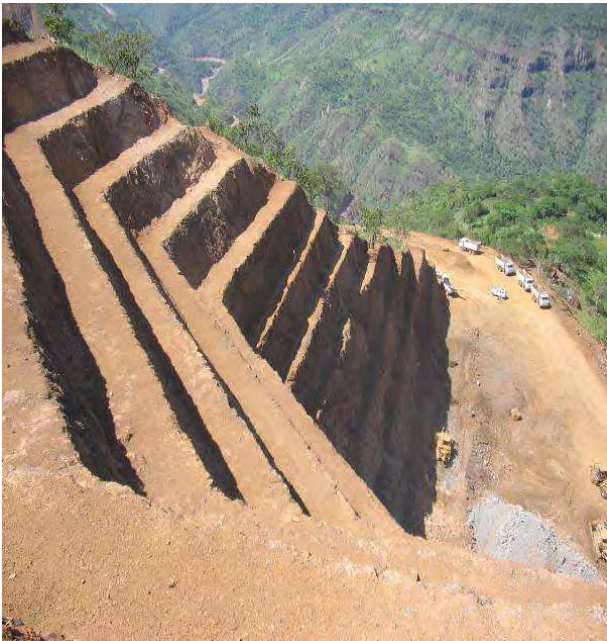
Figure III - 28 Reprofiling and settlement of the Outlet area slopes - Penstock Source: General Contractor photographic doc.
