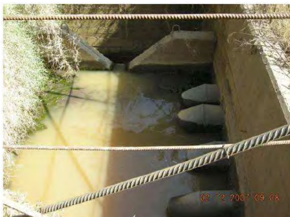
Figure III - 20 Processing unit (sedimentation only) of the waters discharged from the TBM boring activity Source: ELC, December 2007
