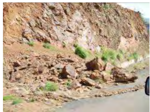
Figure II- 9: Rockfall on the roadway Source: photographic documentation of the evaluation team
