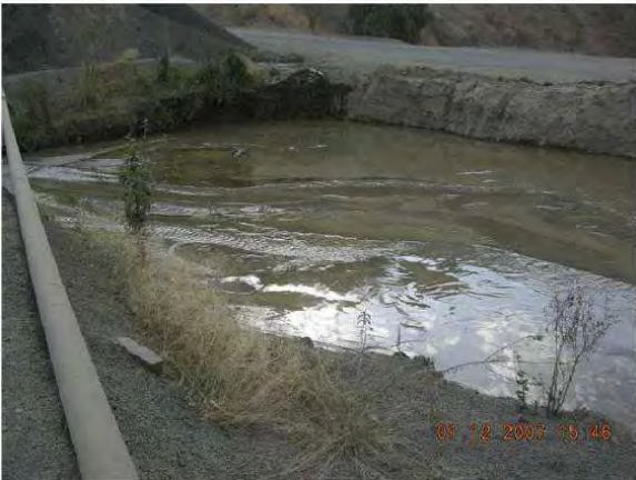
Figure III - 24: Partially soil filled settling basins Source: ELC, December 2007
