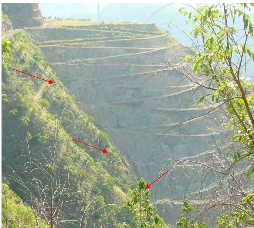
Figure III - 45: "Disposal Area" Outlet side, evidence of badland erosion furrows on the mound Source Evaluation Team photographic doc. 05.2012
