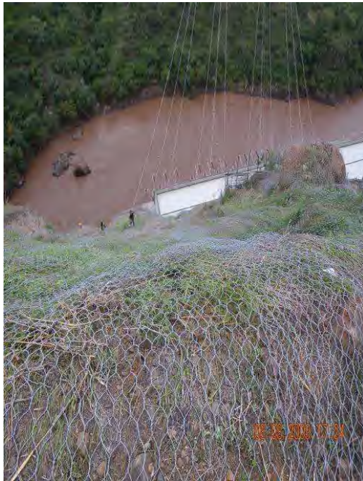
Figure III - 30: Mountainside stabilisation, Power H. area, using wire netting and riveting Source: General Contractor photographic doc., 08.2009
