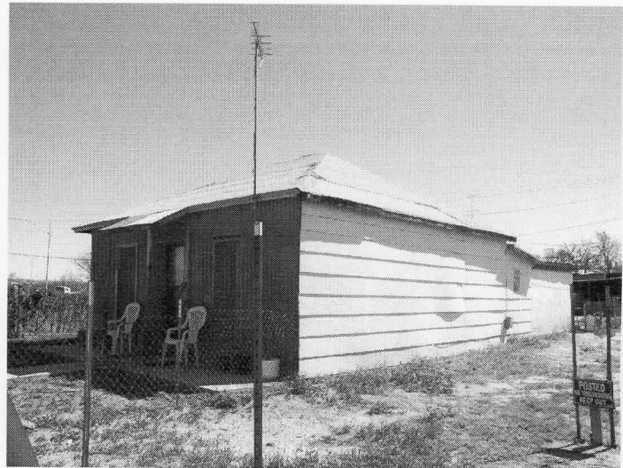
Photo 10. 550 E. Fifth Street. This is a classic pyramidal cottage built in 1930 of stuccoed adobe. The west wall has blue, horizontal, composition siding.
