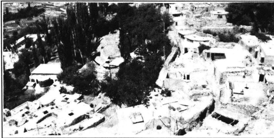
Fig. 5.4 The site after the demolition of the jamat khana building. Photo taken in August 1988.
