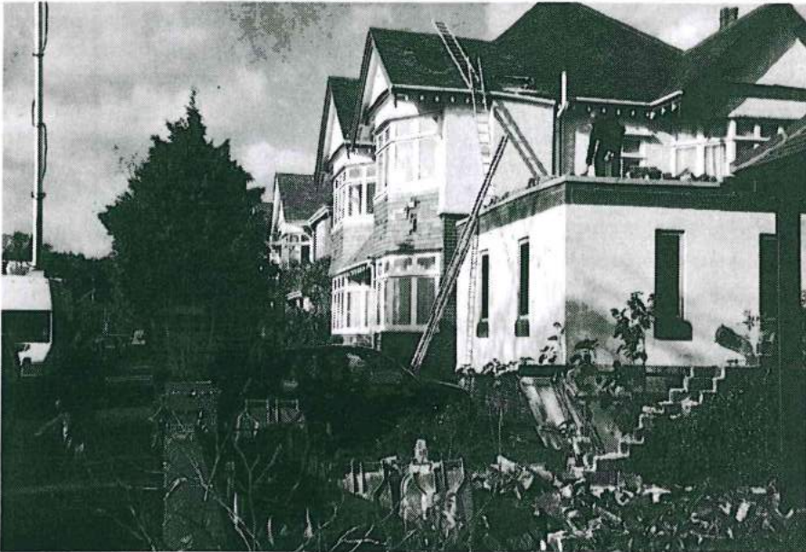
Fig. 2. Looking NW towards 24 Oakmount Avenue. In the background the chimney was removed from No. 24 and deposited next to where the workman is standing. In the foreground a section of the double-skinned wall was brought down in an easterly direction showing the force of the winds (see also Fig. 3)
