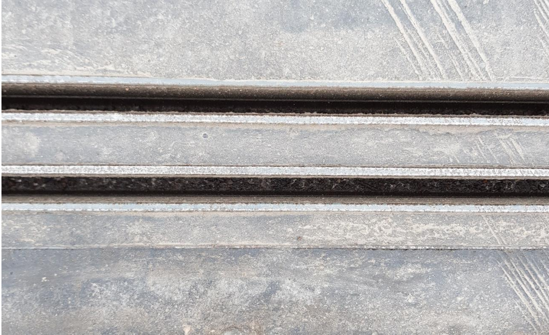
Figure 25: Wear on the ERS conductive rail.
