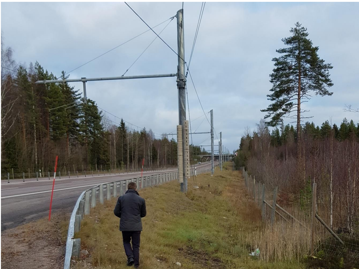
Figure 21: Catenary poles and roadside safety barriers along E16, Sweden.
