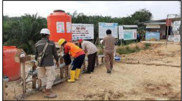
Figure 8.15-2: Hand washing facility on-site
