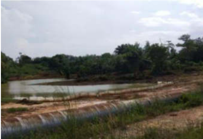
Figure 8.6-4: Silt fence installation to avoid runoff surface during heavy rainfall at water pond area (KP 07)
