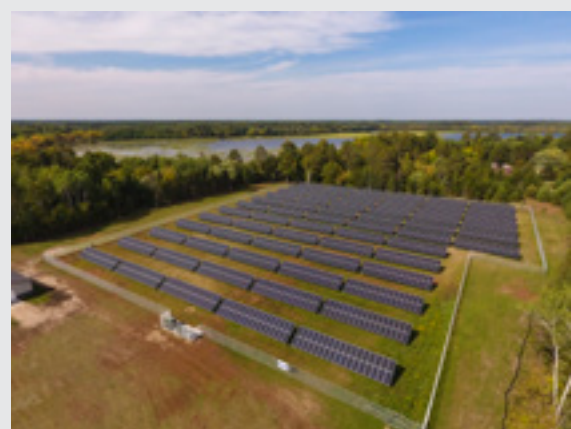
Solar array for Pine River-Backus High School
