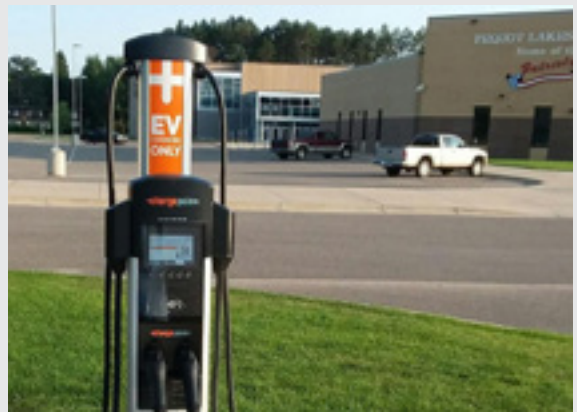
Electric vehicle charging station outside Pequot Lakes School
