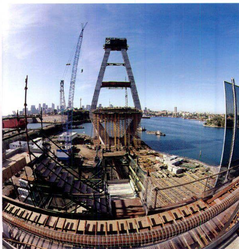
With two 120 metre high towers and a main span of 345 metres, Glebe Island Bridge, Sydney, will be the longest cable-stayed bridge in Australia.
