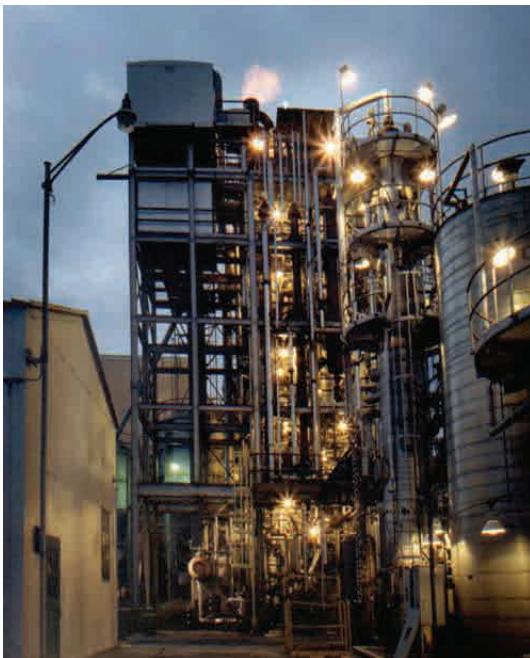
The fixed-bed coal gasification pilot plant at Morgantown by night.
