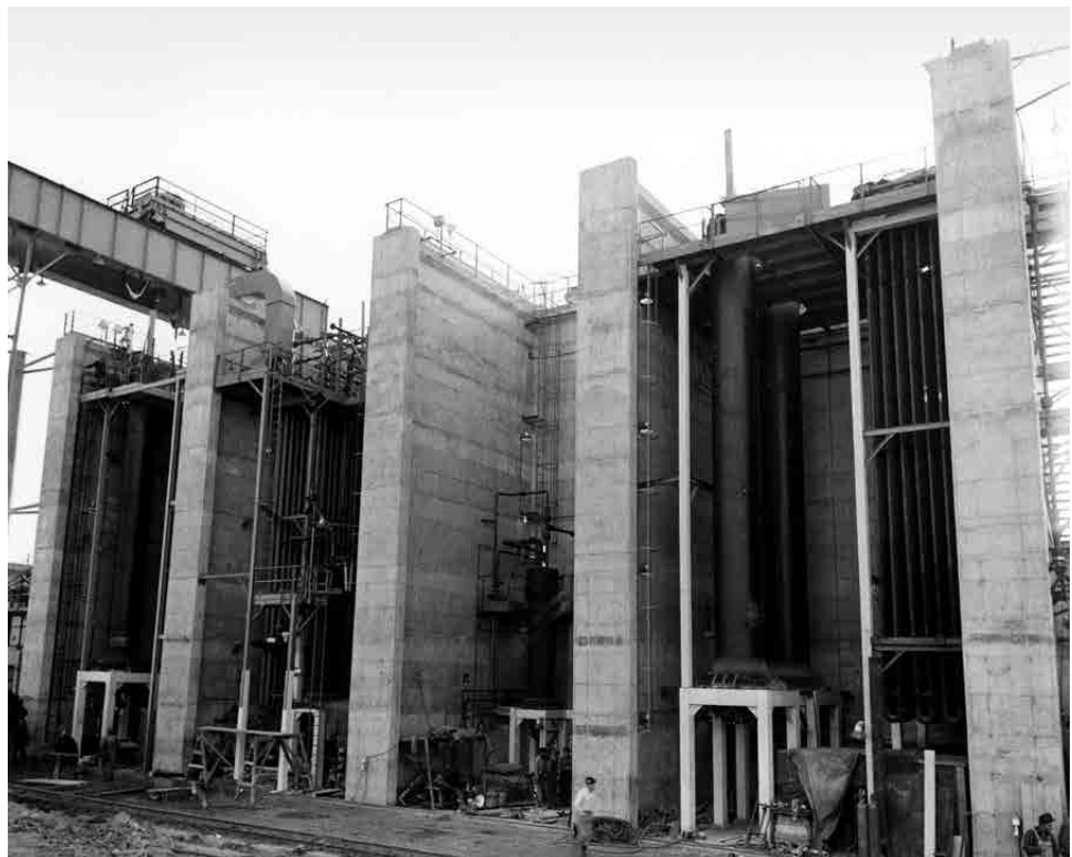
Coal-hydrogenation converter stalls bracketed by thick concrete at the Louisiana demonstration plant. (photo credit: National Archives and Records Administration)
