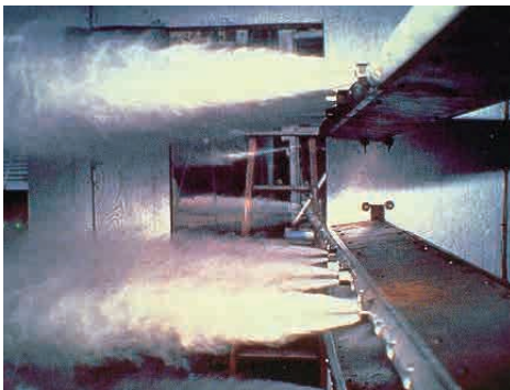
At Edgewater, an important step in the Coolside and LIMB sulfur-removal processes involved spraying the flue gas with mist to humidify it.
