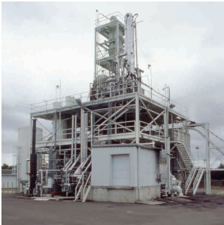
Plant designed to extract oil from wood waste materials from the lumber industry, 1977.
