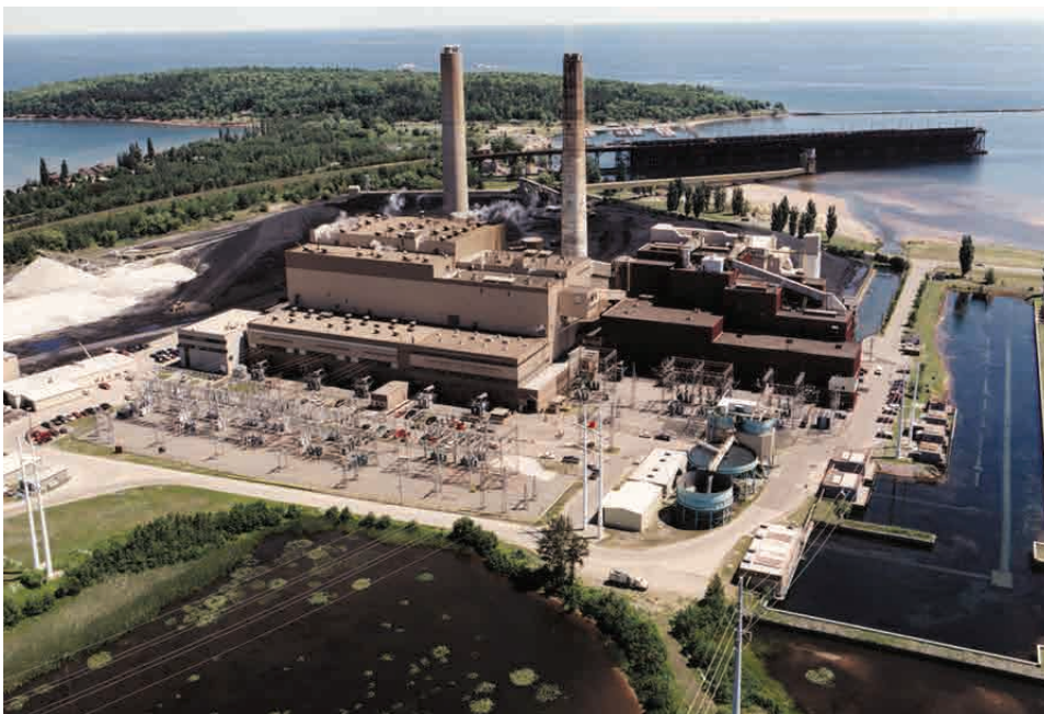
Presque Isle Power Plant in Marquette, Michigan, where the TOXECON mercury-removal technology was tested.
