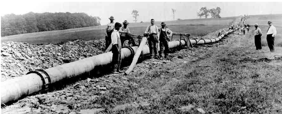
A natural-gas pipeline under construction in 1922. Advances in pipeline technology during the 1920s and the 1930s made long-distance distribution of natural gas to American towns and cities possible.
