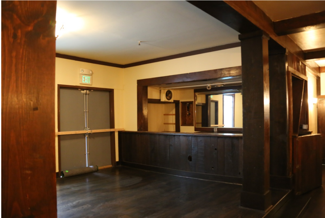
Raised area in rear dining room, view southeast. Not heavy timber framing at left and right.
