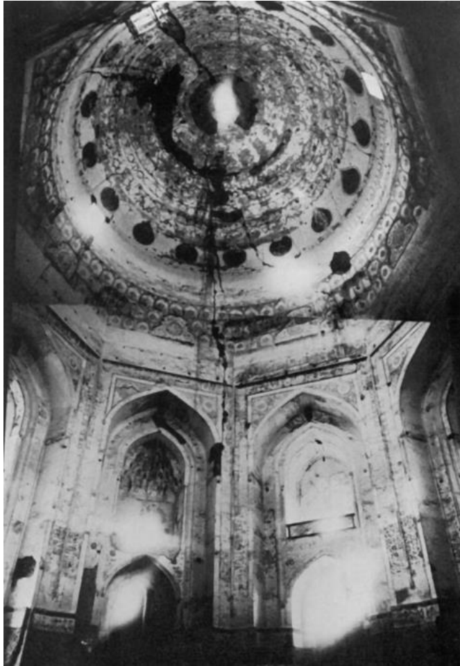
Figure 4: ca 1970's image of the interior of the Soltaniyeh dome revealing distinctive vertical cracking patterns associated with outward movements of support walls. This image comes directly out of Piero Sanpaolesi's paper, "La cupola di Santa Maria del Fiore ed il mausoleo di Soltanieh. Rapporti di forma e struttura fra la cupola del Duomo di Firenze ed il mausoleo del Ilkhan Ulgiaitu a Soltanieh" (1972)
