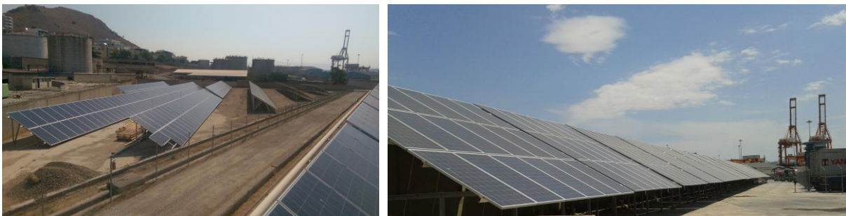
Figure 8. PV panels installed along a wall and on the ground.
