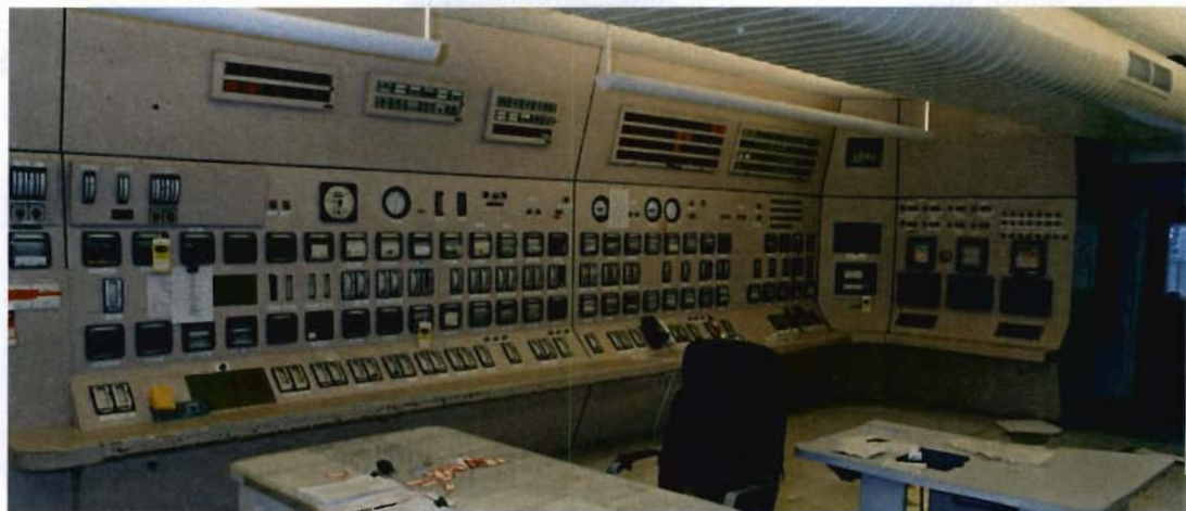
Figure 2.13 Photograph of GPI Pneumatic Control Panel (taken after the Bailey equipment was removed for examination)
