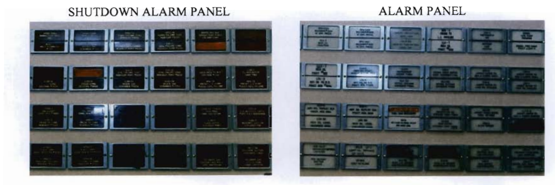
Figure 2.17 Photograph of GP1 alarm panels
