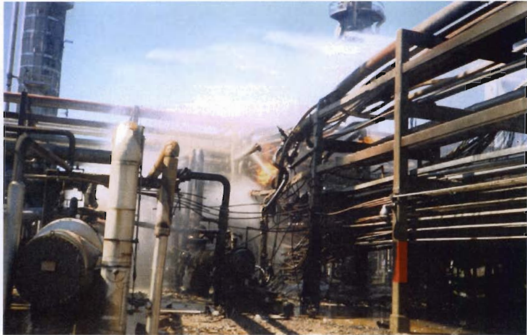
Figure 7.16 Photograph taken at approximately 14:45 pm, 26 September, showing seats of fire in Kings Cross piperack
