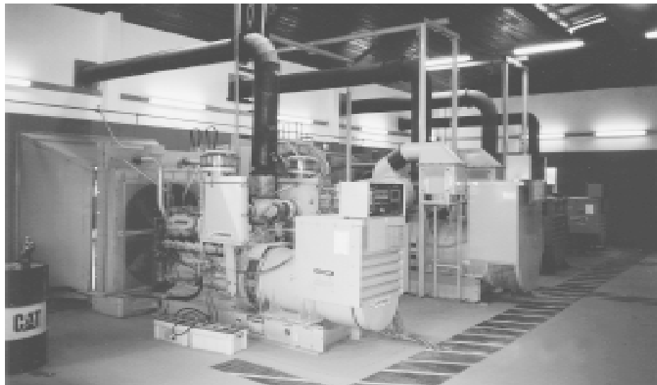
Diesel power plants at Gruenau South Menno that will soon be replaced by the arrival of Federal power from the Itapou power station on the Parana River.
