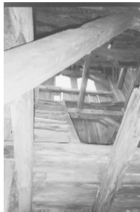
A photograph of the wood structure inside the old wind mill building. The basic frame of the building consisted of four huge beams 20 inches square. Each beam had a wooden inscription carved into it. One of them read: "Anno 1792 is dieser Thurm gebaut, der Bauherr ist gewesen, Isaak Quapp, Schulz auf Neunhuben" ("The tower was built in 1792, the construction supervisor was Isaac Quapp, Mayor of Neunhuben").
