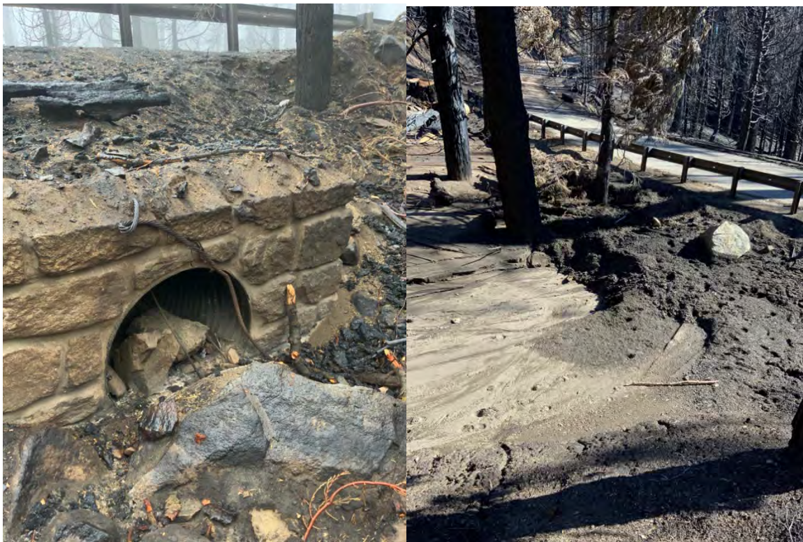
Figure 1. A culvert up the road from Red Fir Maintenance facility before and after the Oct 25 storm
