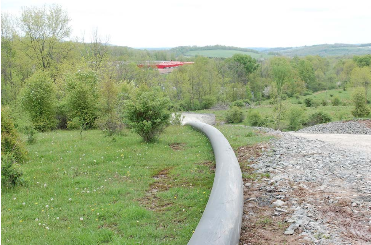
Photo 5.21 Water pipeline from Fortuna central freshwater impoundments, Troy PA. Source: NYS DEC 2009.
