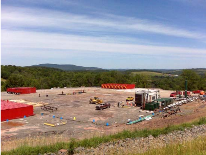
Photo 5.26 Fortuna multi-well pad after hydraulic fracturing of three wells and removal of most hydraulic fracturing equipment. Production equipment for wells on right side of photo. Source: Fortuna Energy, July, 2009.
