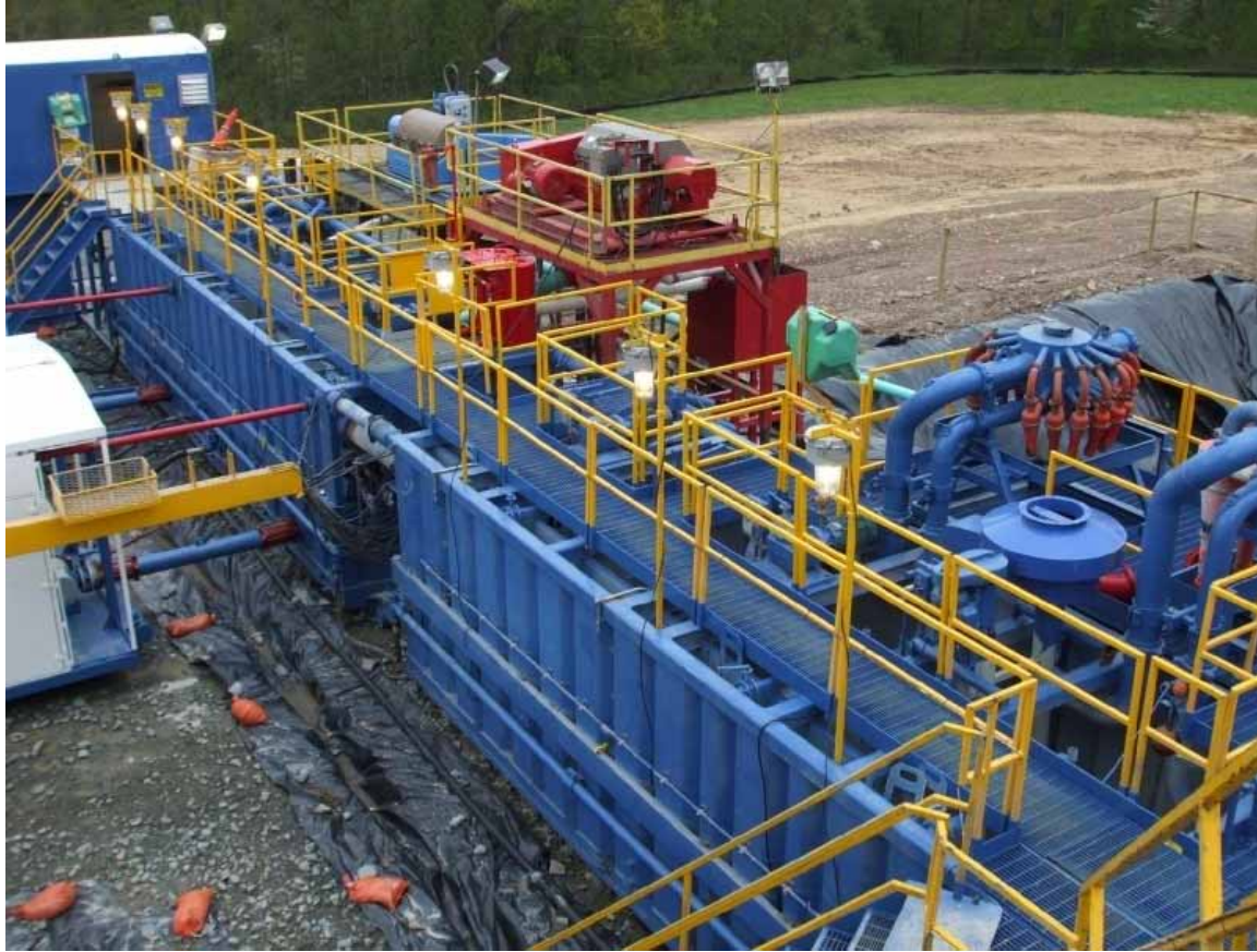
Photo 5.16 - Drilling rig mud system (blue tanks)
