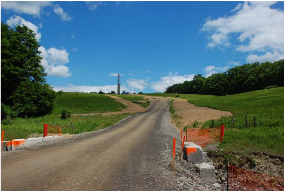
Photo 5.1 Access road and erosion/sedimentation controls, Salo 1, Barton, Tioga County NY. Photo taken during drilling phase. This access road is approximately 1,400 feet long. Road width averages 22 feet wide, 28 feet wide at creek crossing (foreground). Width including drainage ditches is approximately 27 feet. Source: NYS DEC 2007.
