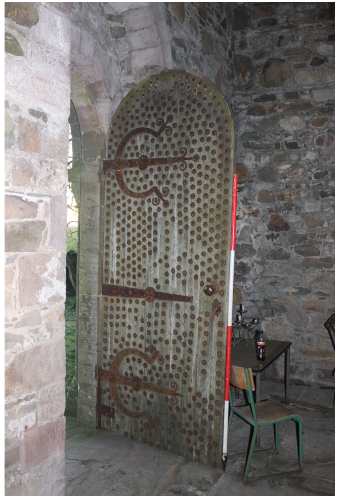
Figure 60: detail of the door F01 in the south wall of the Nave, from the north-east
