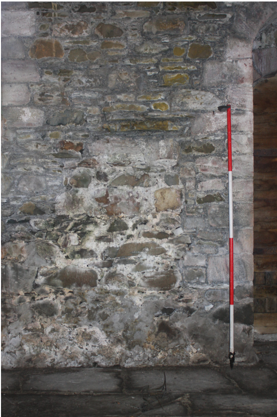
Figure 74: detail of recessed/ blocked feature F10 in the south wall of the Chancel
