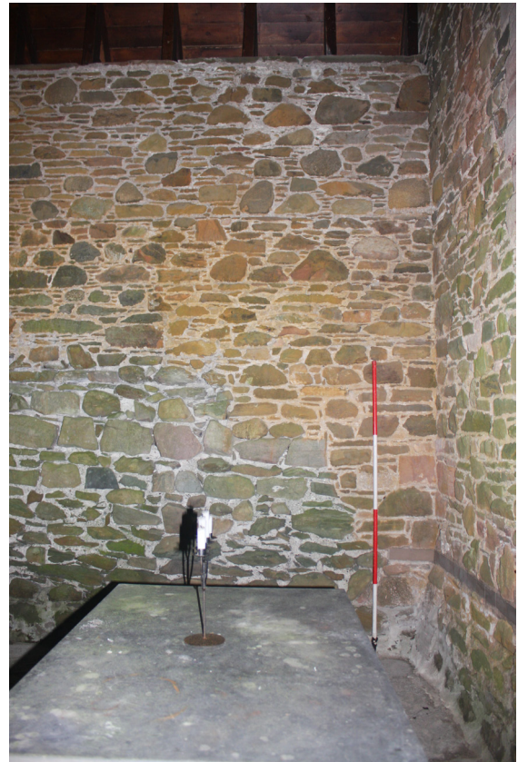
Figure 75: general view of the north wall, showing the phase line between the original and rebuilt wall, from the south
