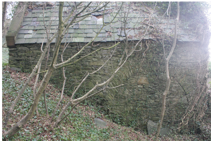
Figure 88: detail of the north elevation of the Chancel showing the blocked arch, from the north
