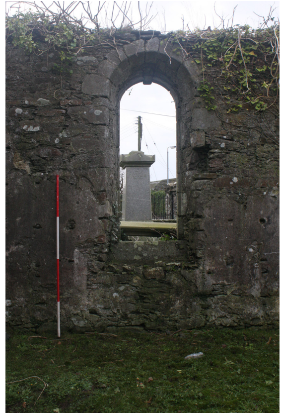
Figure 126: detail of round-headed window on the south wall (interior) from the north
