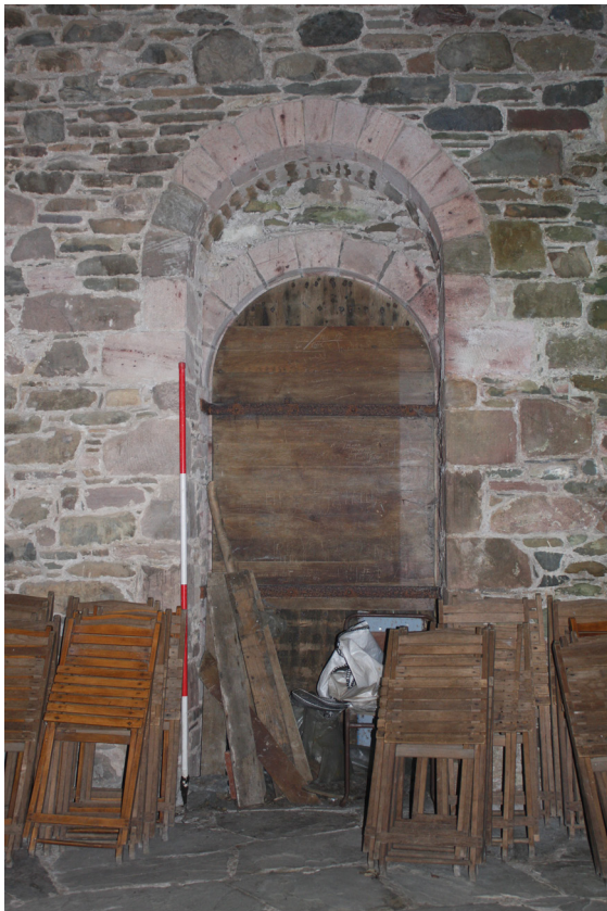
Figure 62: detail of door F03 in the north elevation of the Nave, from the south
