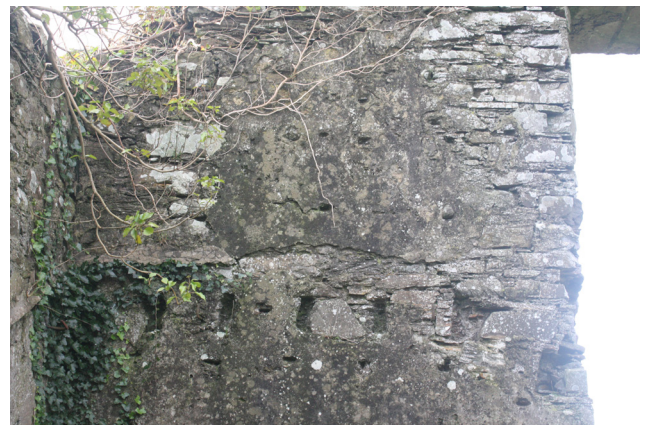
Figure 128: detail of beam slots to the south side of the west gable (interior) from the east
