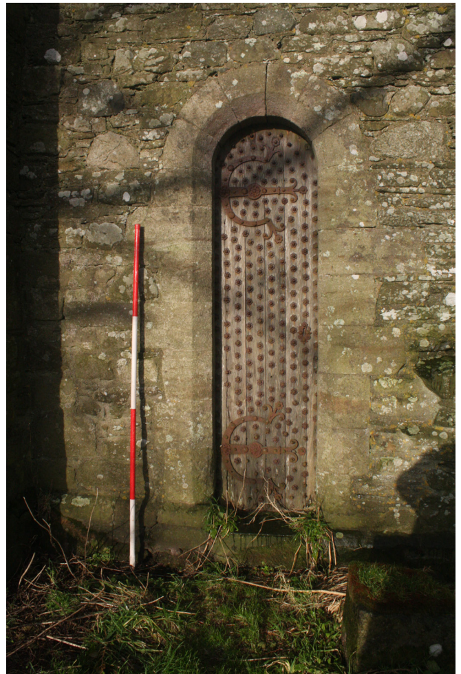
Figure 56: detail of the door to the Chancel (F09) to the east side of the south elevation
