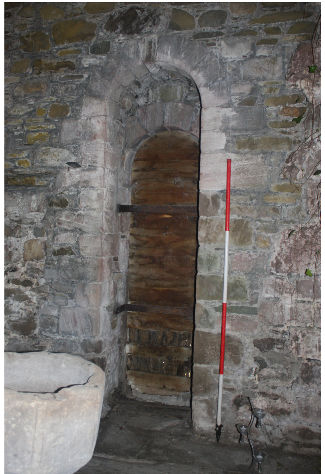
Figure 72: detail of door F09 in the south wall of the Chancel, from the north-west
