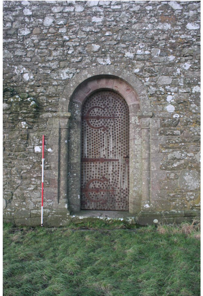
Figure 50: Detail of the door to the Nave (F01) to the west side of the south elevation SE.
