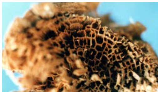
Figure 147. Advanced decay. Honeycomb appearance of decayed wood.
