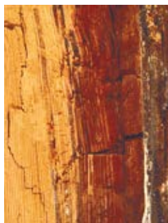
Figure 254. Advanced decay of Douglas-fir wood.
