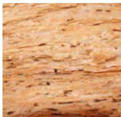
Figure 149. Advanced decay symptoms. Black flecks and stringy appearance are distinguishing features.
