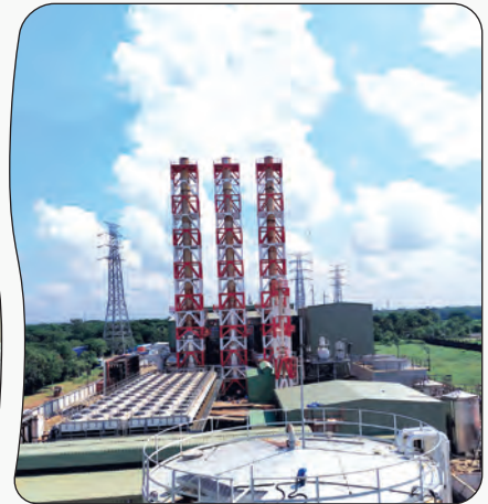
Potiya 54 MW Power Plant
