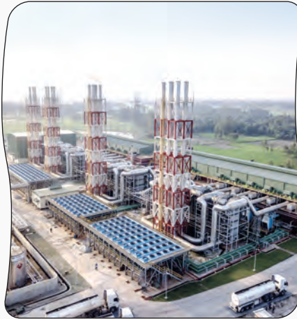
Rangpur 113 MW Power Plant
