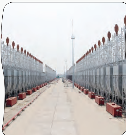
Baghabari 200 MW Power Plant
