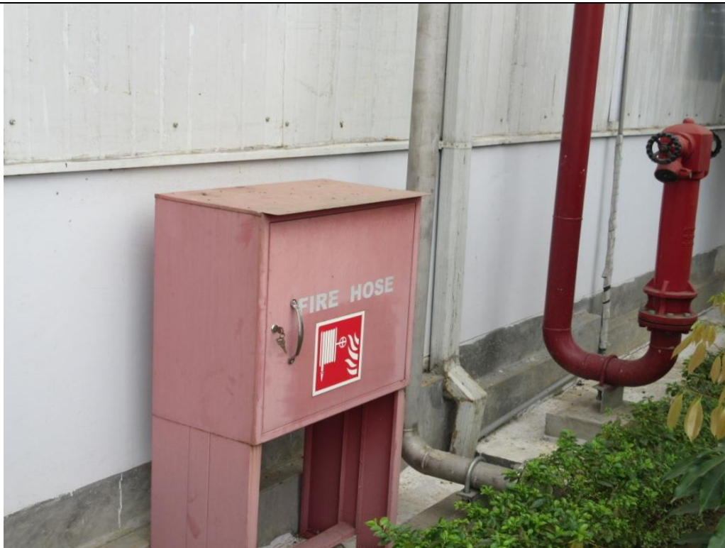
Photograph: Different types of fire-fighting arrangement
