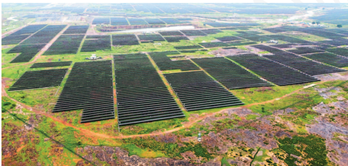
750 MW, Rewa Ultra Mega Solar power plant in Gurh, Rewa, Madhya Pradesh (India).
