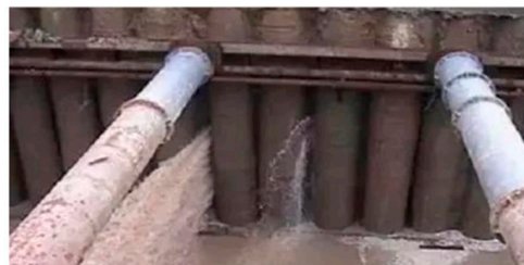
(c) Poor quality of water stop curtain
