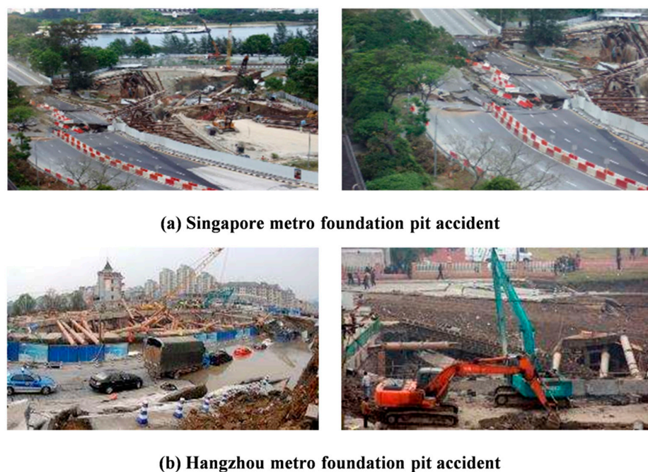
Figure 6. Metro foundation pit accident.
