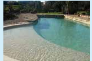
Salt water & UV water treatment system
