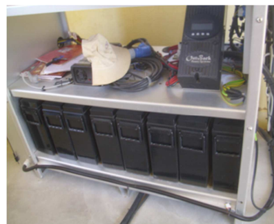
Figure 55: Batteries de 24 V 100 Ah
