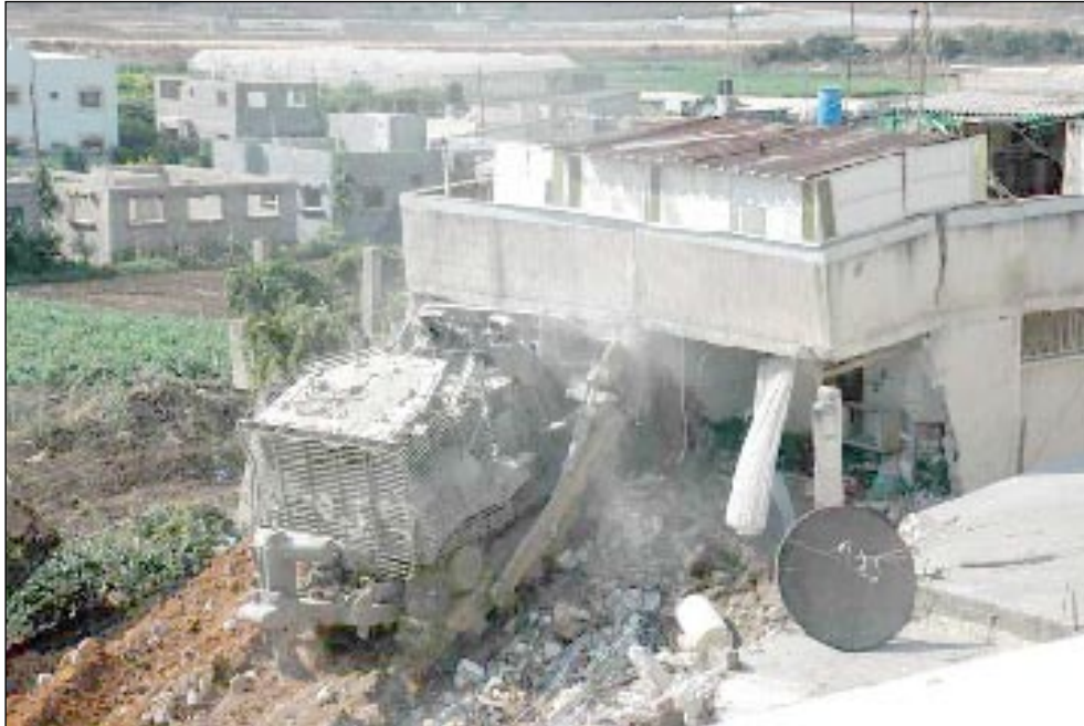
Home demolition in al-Nuqar (Qalqilya district) on 29 August 2007 (Badil).
