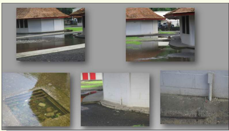
ASDOE Schools Electrical Common Problems of 10 Schools
