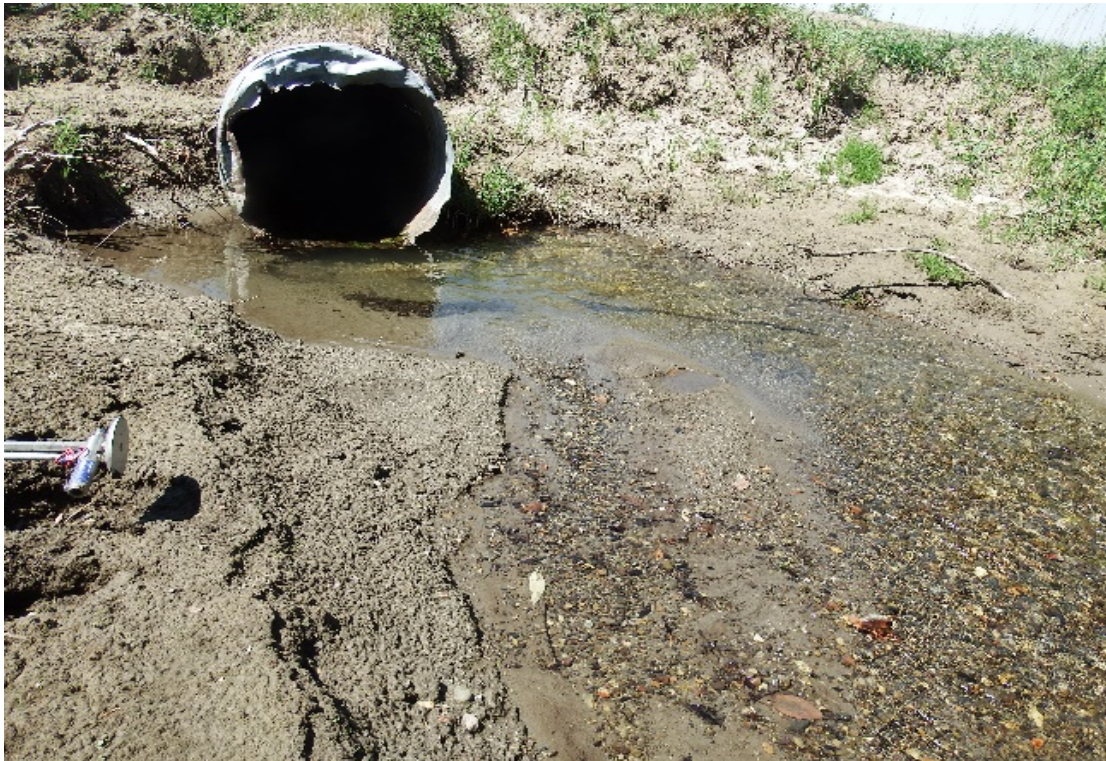
Figure 6-4. Culvert and siltation in Jones Creek about two miles downstream of the South Valley Road crossing
